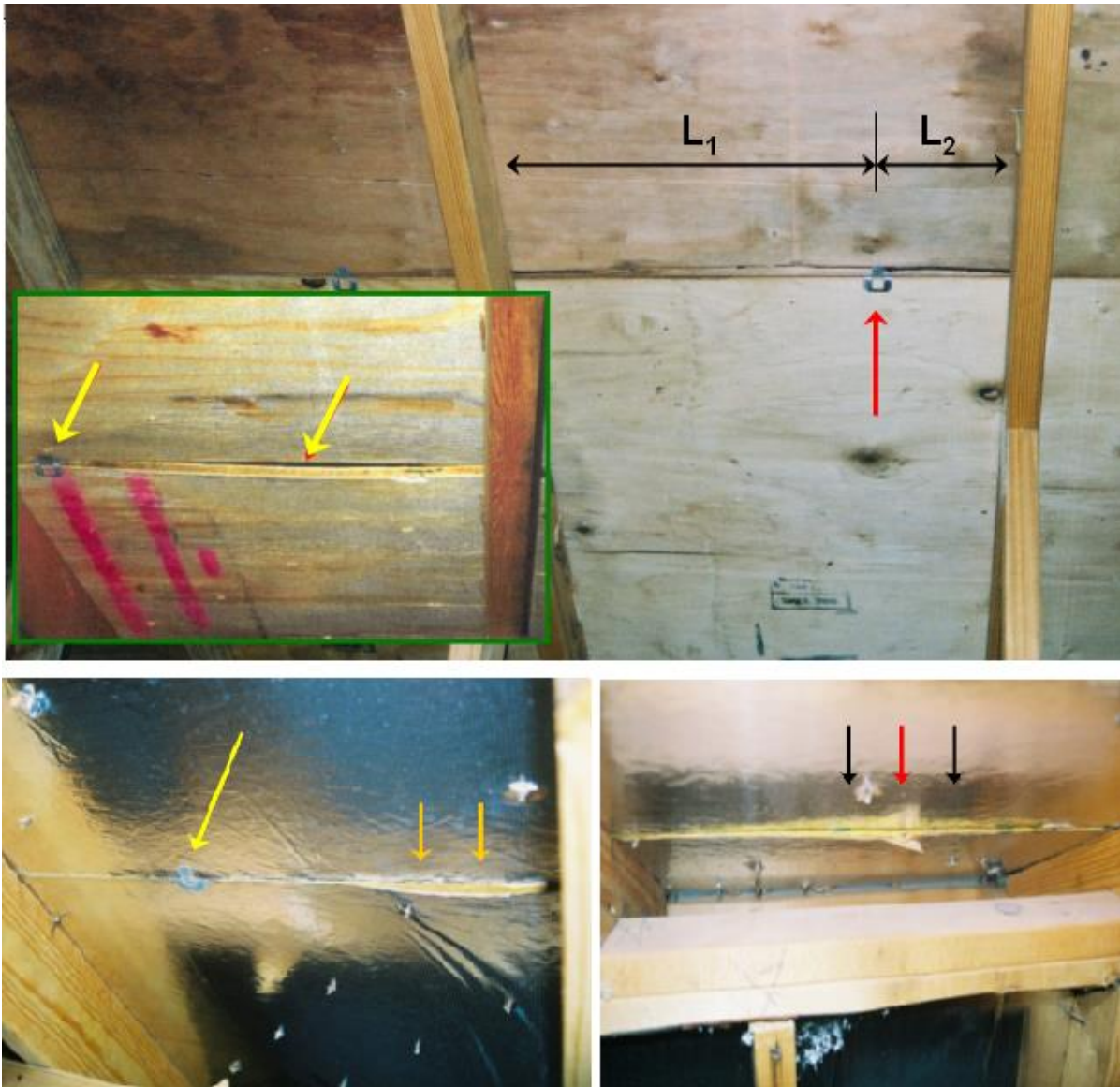
Figure 2. Panel edge clip (H-clip) installation errors – misplaced and/or missing edge clips
